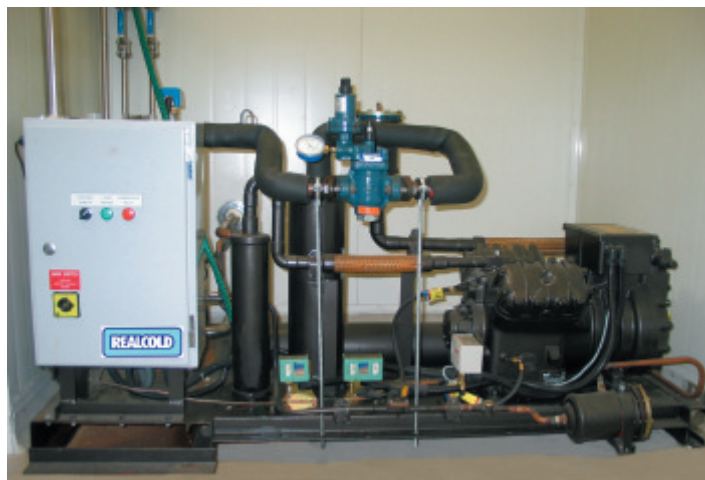
A purpose-built water chiller in a working/industrial environment.
